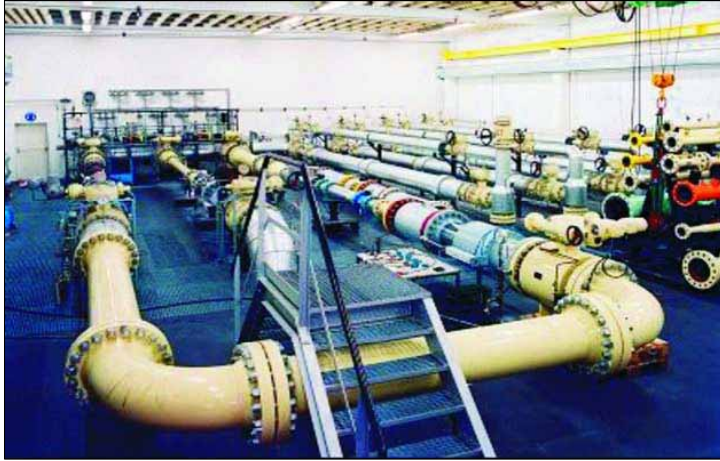
Figure 2: pigsar™: Working standards and meter test sections
