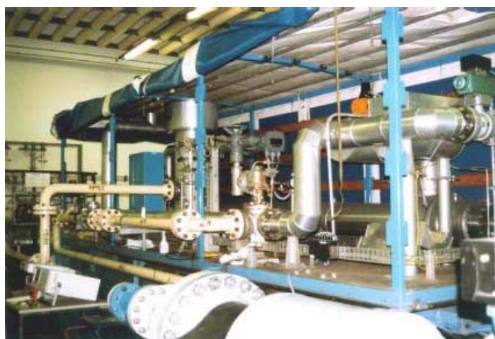
Figure 6. Photo of high pressure piston prover (HPPP) mounted on trailer with reference meter
