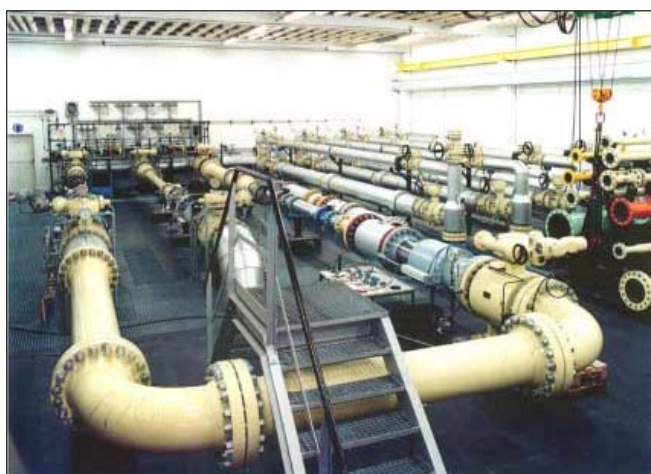
Figure 2. Photo of PIGSAR™. On left side you can see the working section for meters under test and on right side the working standard section.
